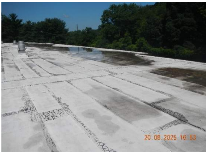
Photo 3 – Overview of lower roof area covered in ponding water.
