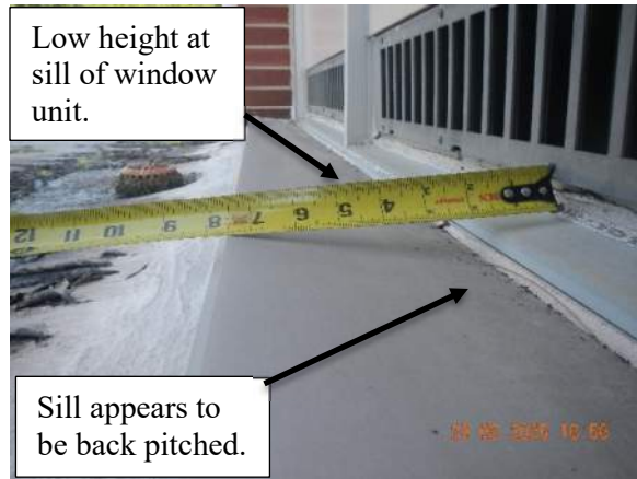
Photo 9 – Low flashing heights at window units on the lower roof.
