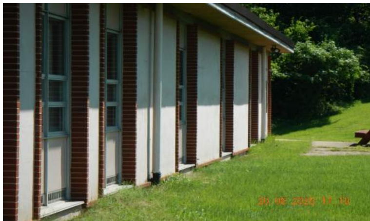
Photo 17 – Typical drain leaders from roof drains. The drains are not part of an internal stormwater system.
